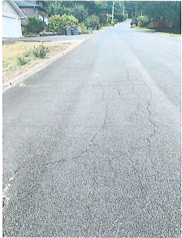
2. More cracking from foundation under roadway unsettled due to excessive water run-off on street.
