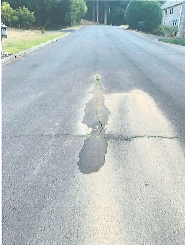
1. Across From Mike Brackenbrough Property (Water on Roadway 24/7 due to failure/shifting roadway water pipe or sewer leak).
