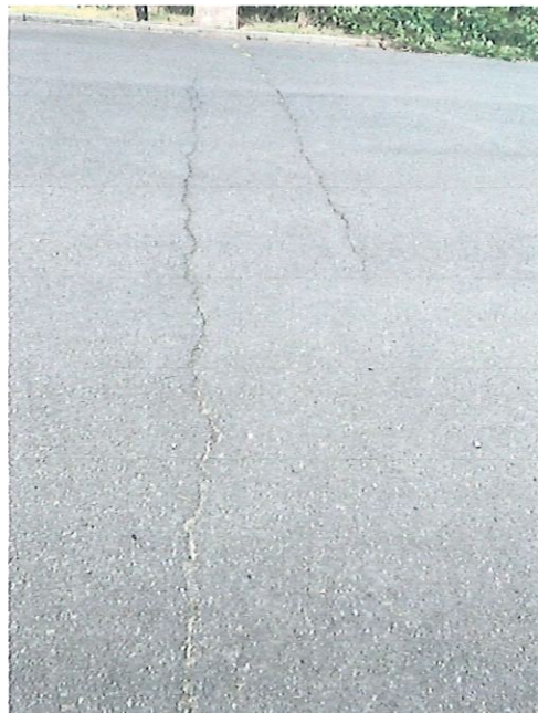
5. Horizontal cracks in roadway due to failure of culvert and shifting of earth due to excessive yearly winter run-off
