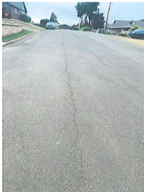
6. Looking west on Aldercrest in front of Boat's House, more visible cracking in pavement which extends to the corner.
